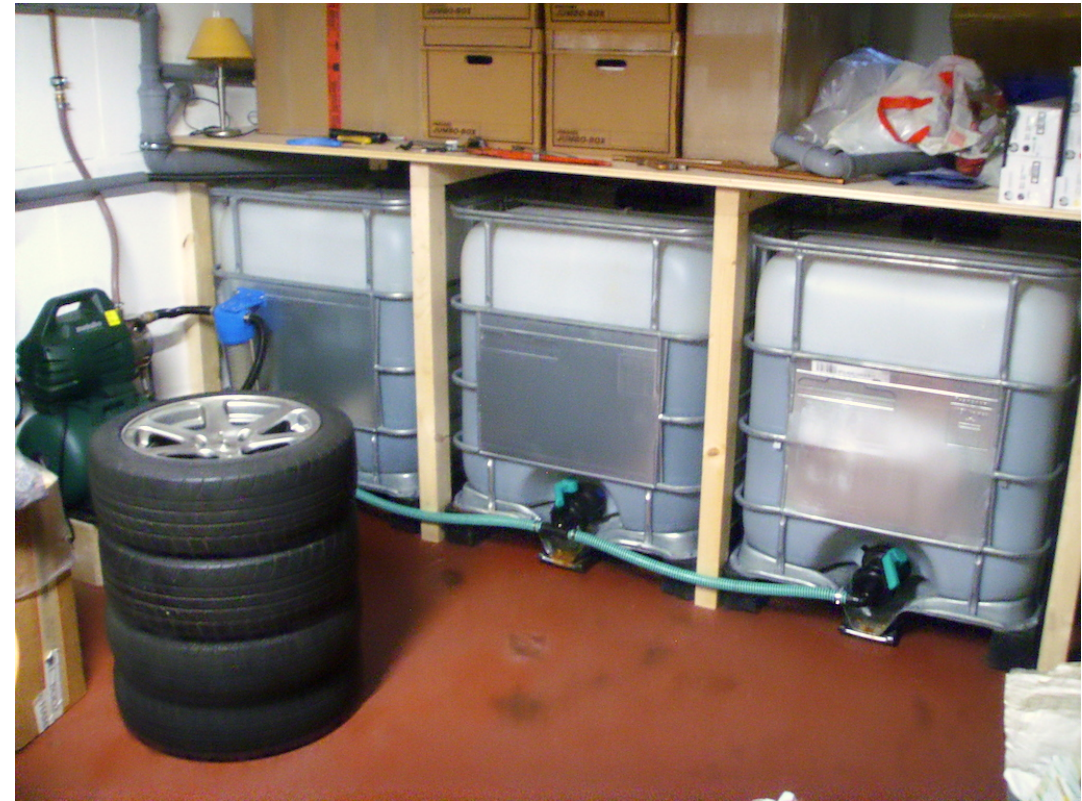
Ultrasonic distance measuring sensor to measure the filling level of rainwater tanks
